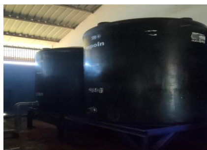
Gambar 3 Raw water tank
